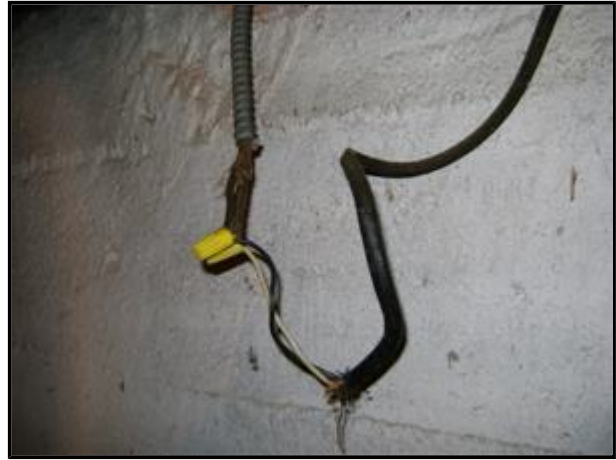
7.3 Picture 2 Open wire splice in basement.
