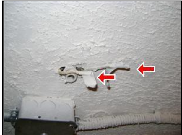
7.3 Picture 4 Cut/taped wires in basement ceiling (live).
