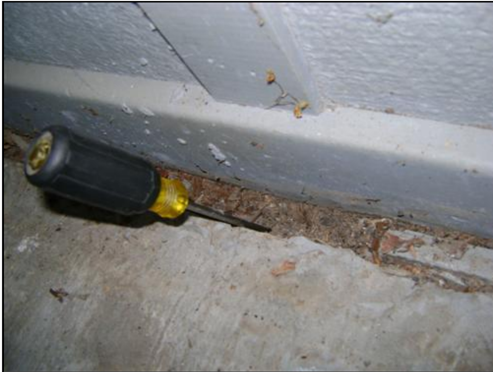
3.1 Picture 1 Deteriorated sill in garage.
