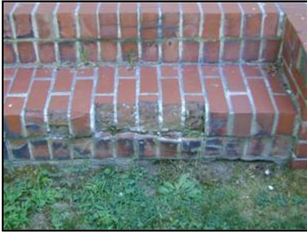
2.3 Picture 1 Deteriorated front steps.
