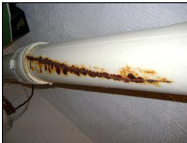
6.0 Picture 2 Cracked waste line in basement.
